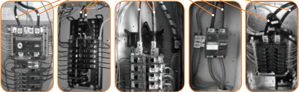
Examples of main cables
